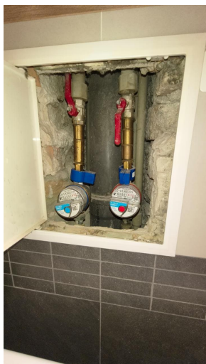
B07 Water connections, valves and meters in the access opening.
