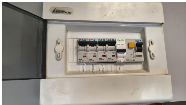
H03 New electrical distribution board.
